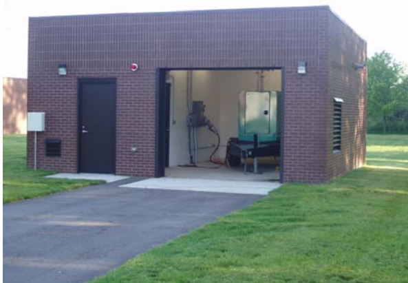
Control Building & Portable Generator
