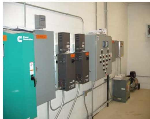
Control Room with Control Panels
