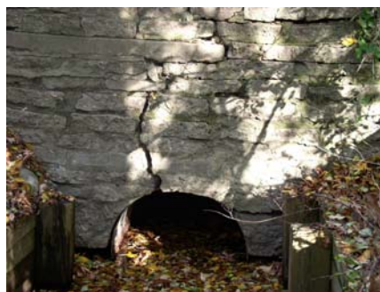
Previous Deteriorated Headwall and Undersized Culvert
