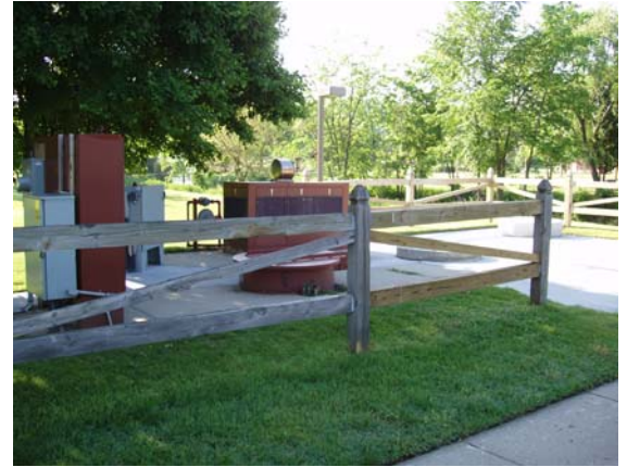
Canal Avenue Lift Station
